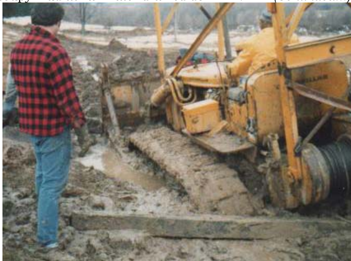
The D-6 has met its match in rain-saturated, semi-frozen ground, and it'll be a while before more work gets done.
