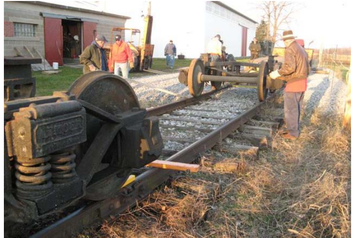
One down and one on the way...the work car trucks are off the trailer and reporting for duty.
