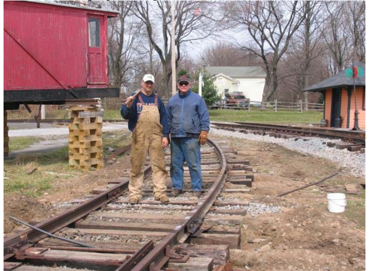
Charlie Lowe and Bob Achilles pause to survey their handiwork on the main barn lead. Charles E. Lowe photo
