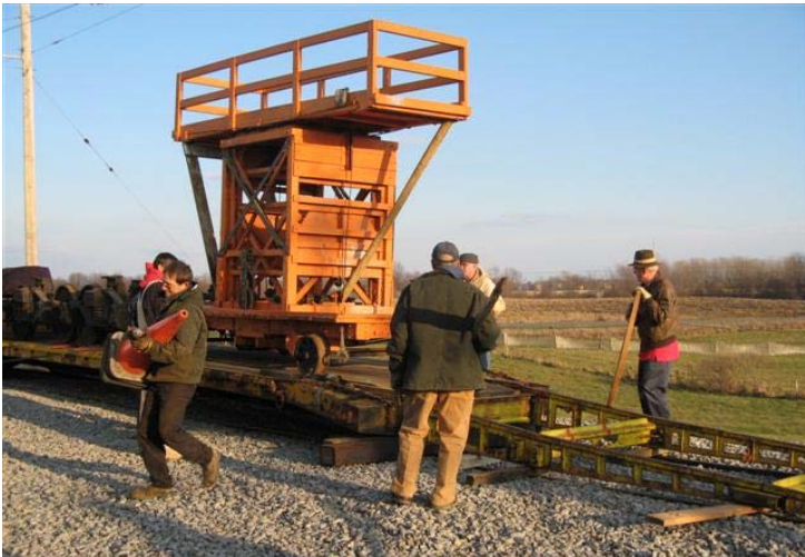
The tower car is ready to come down the ramp...all we need to do is make sure it doesn't get away from us.
